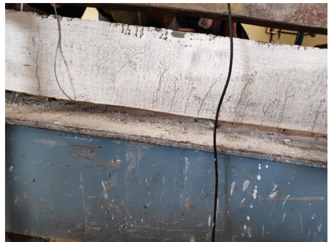
FIG 10 CRACKS ON BEAM
